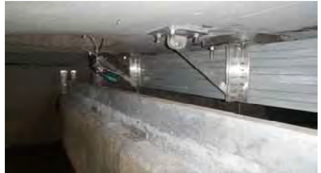
Floatables control underflow baffle installed behind the existing SOM01A overflow weir
