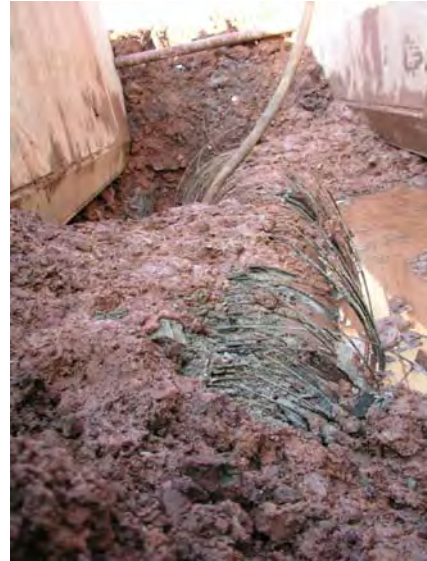
Example of a brittle wire failure
