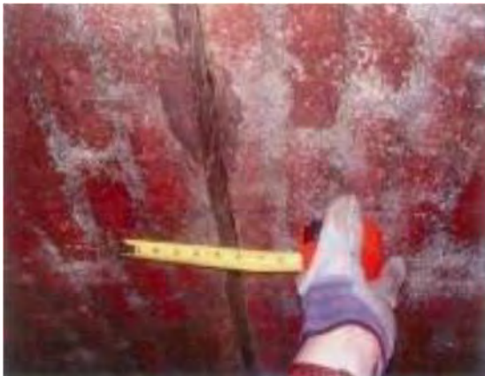
Crack in Rosemary Brook Siphon
