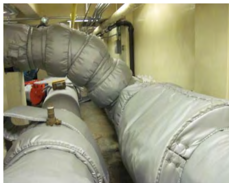
Insulation of Water Piping
