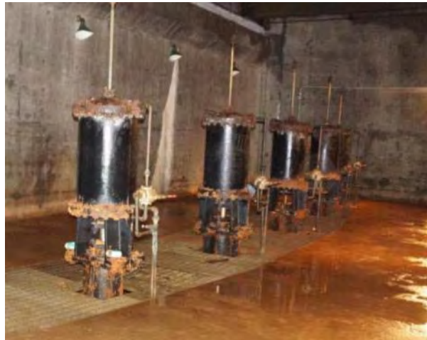
Shaft 7 valve actuators
