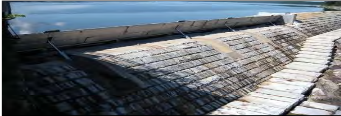
Wachusett Spillway Crest Gate
