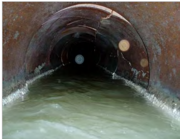
Example of sewer needing rehabilitation
