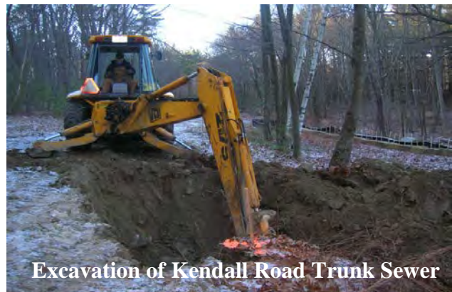
Failed Trunk Sewer off Kendall Road
