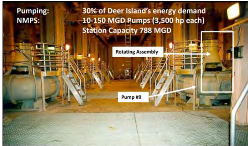
Figure 12: DITP North Main Pump Station - Pump 9
