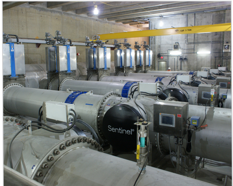
Ultraviolet light reactor units recently installed at MWRA's Carroll Water Treatment Plant in Marlborough. The Quabbin facility will be equipped with three, 24-inch Sentinel UV Light Reactor units manufactured by Calgon Carbon Corporation.
