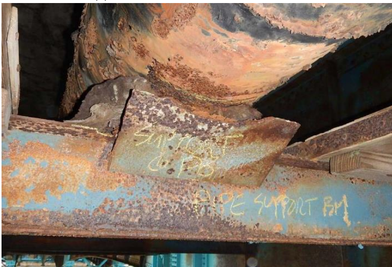
Figure 6 – Typical Deteriorated Pipe Support and Support Beams
