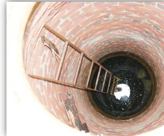
Shaft 7D connecting pipe air valve chamber
