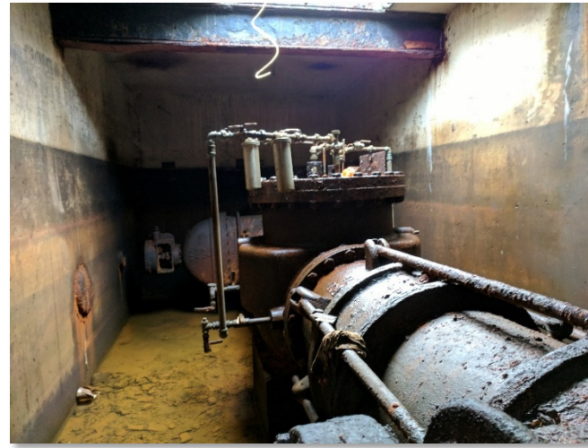
Pressure Reducing Valve Improvements
