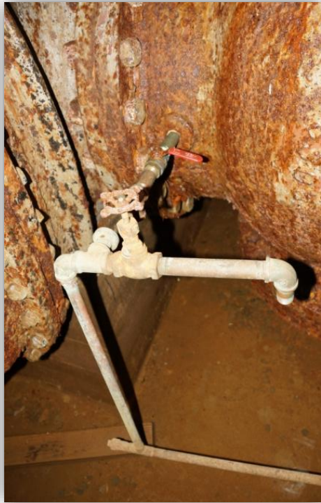
Control piping at Shaft 8
