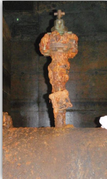
Air valve at Shaft 9A
