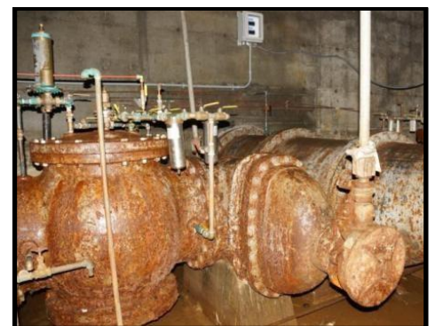
Tunnel valves in need of repair
