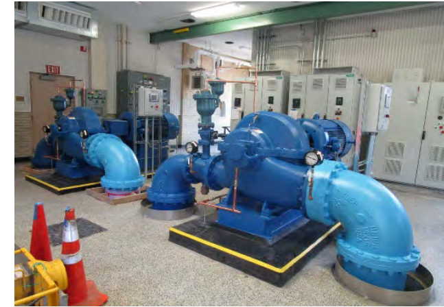
New Pumps at Commonwealth Avenue
