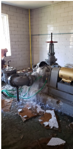
Linden Street Pump Station Wakefield 4/27/21
