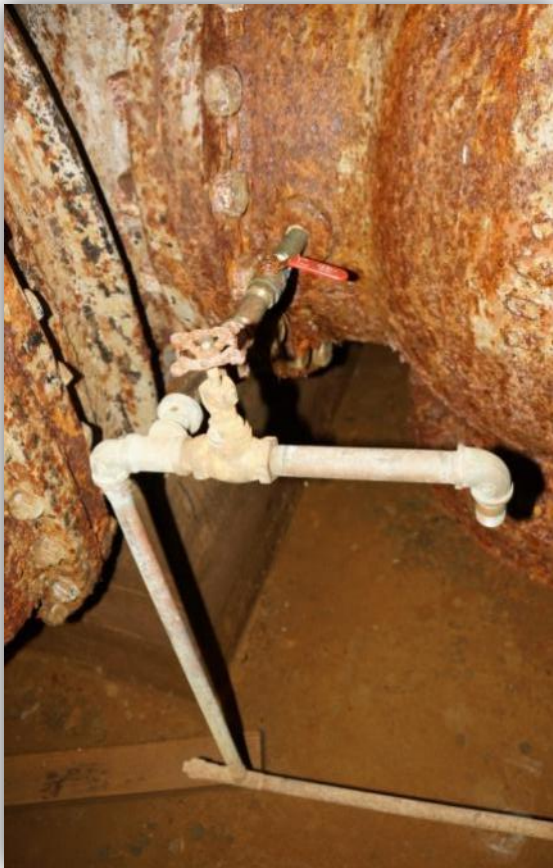
Control piping at Shaft 8
