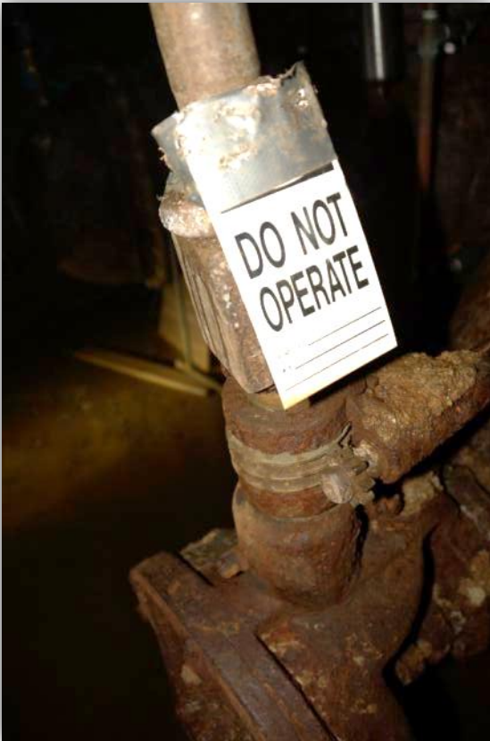
Shaft 8 PRV Chamber
