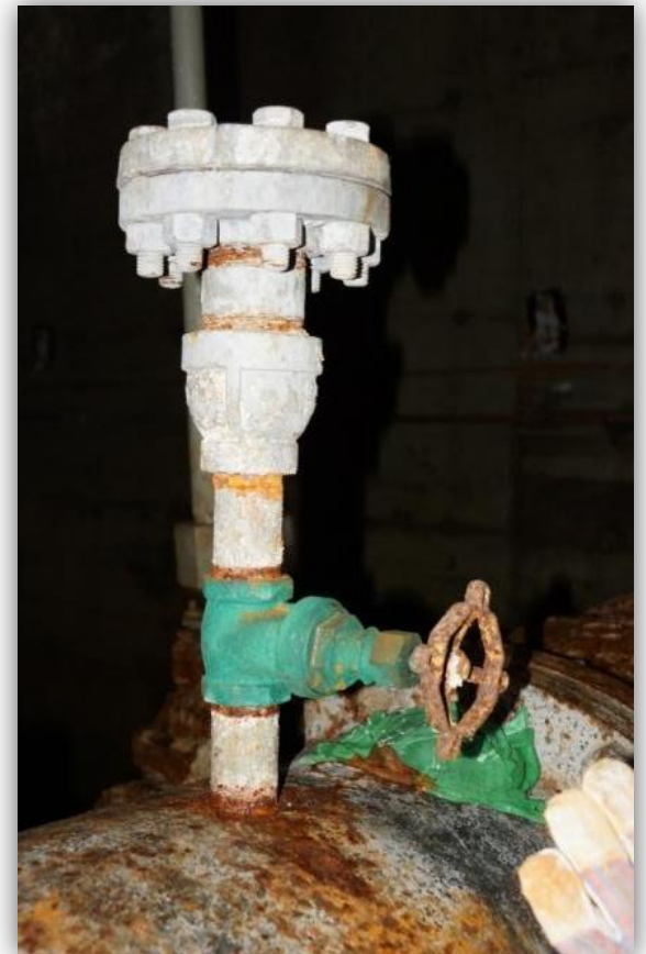
Shaft 8 PRV Chamber
