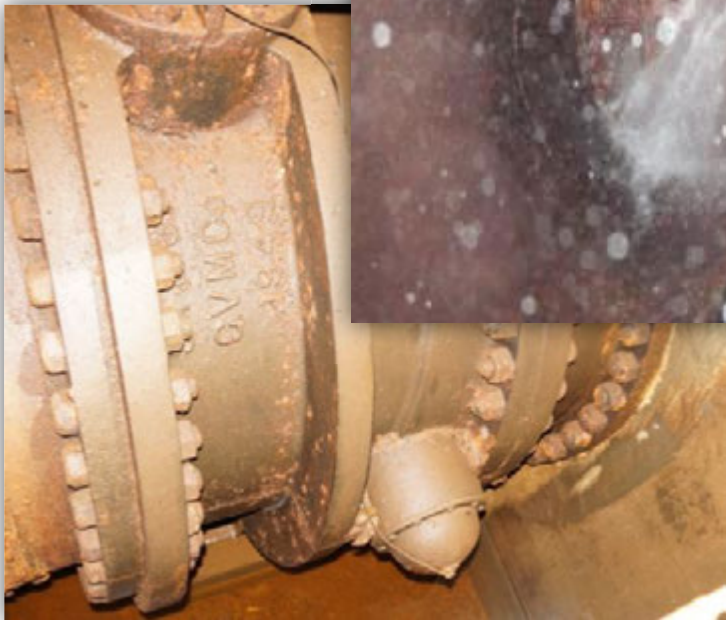
54-inch Shaft 7 Valve
