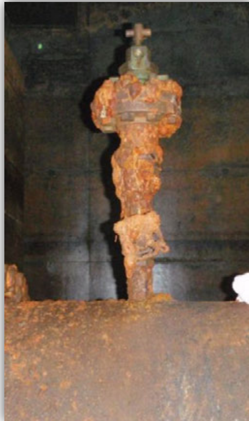
Air valve at Shaft 9A
