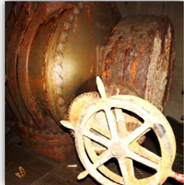
Cone Valve at Shaft 7B
