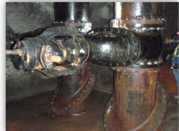
20-inch Shaft 7 Valve
