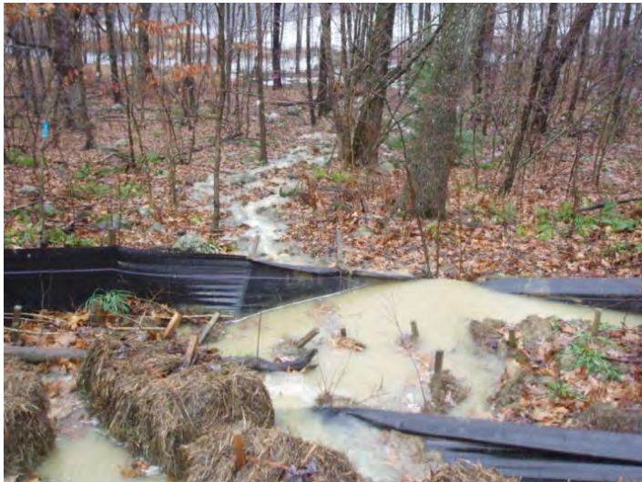
Overwhelmed erosion controls with sediments flowing through wetland to Moulton Pond, November 2008.
