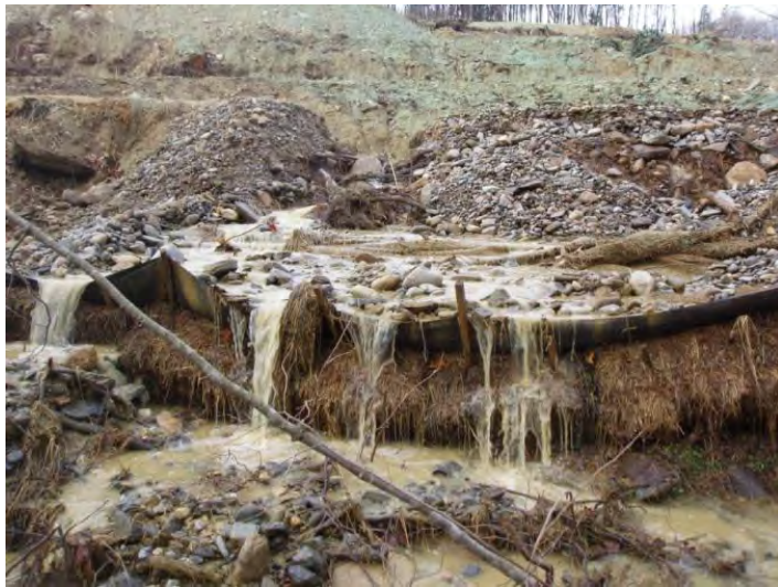
One of the first erosion events, November 2006
