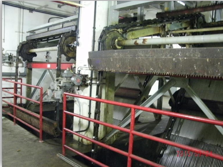
Catenary Bar Screens to be Replaced
