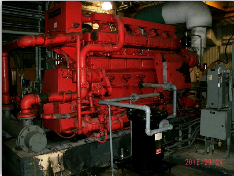
Storm Pump Engine to be Replaced
