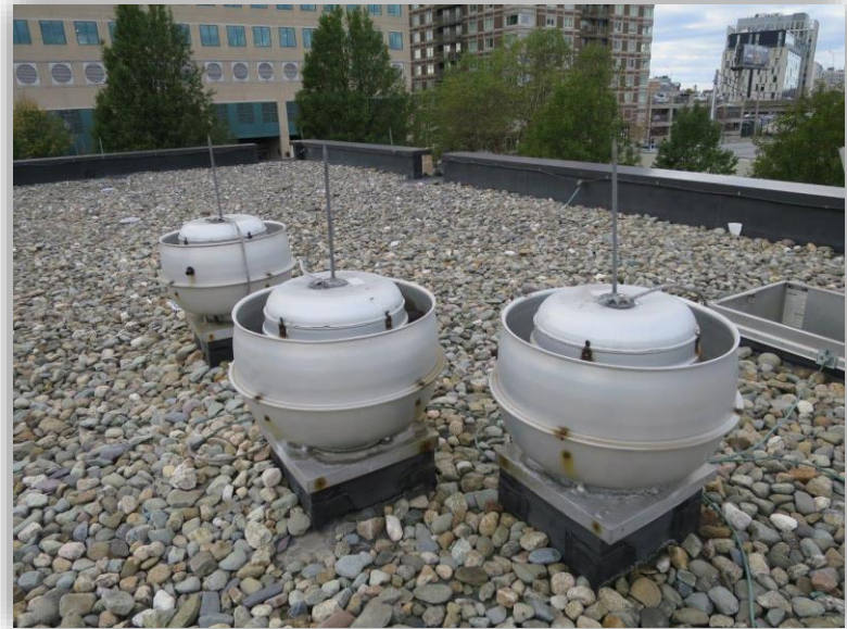
Replacement of Chemical Building Roof and Installation of Chemical Tank Access Hatches
