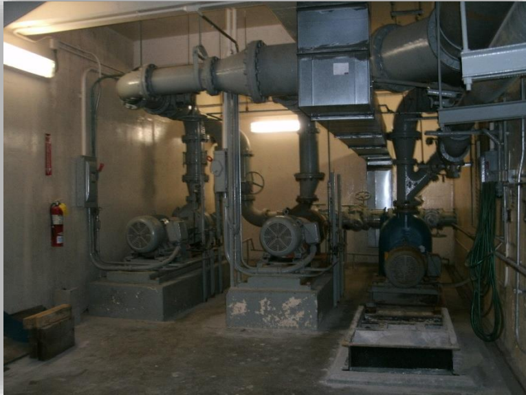
Dry Weather and Dewatering Pumps to be Replaced
