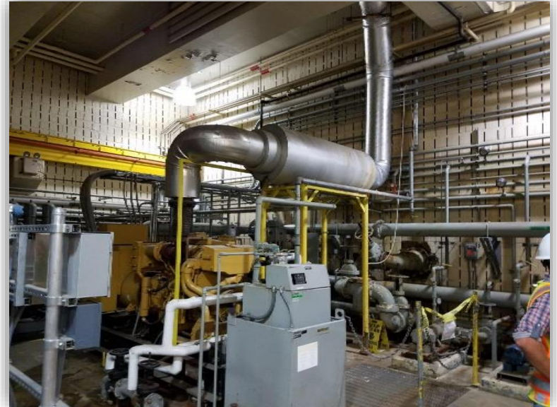
Generator to be Replaced
