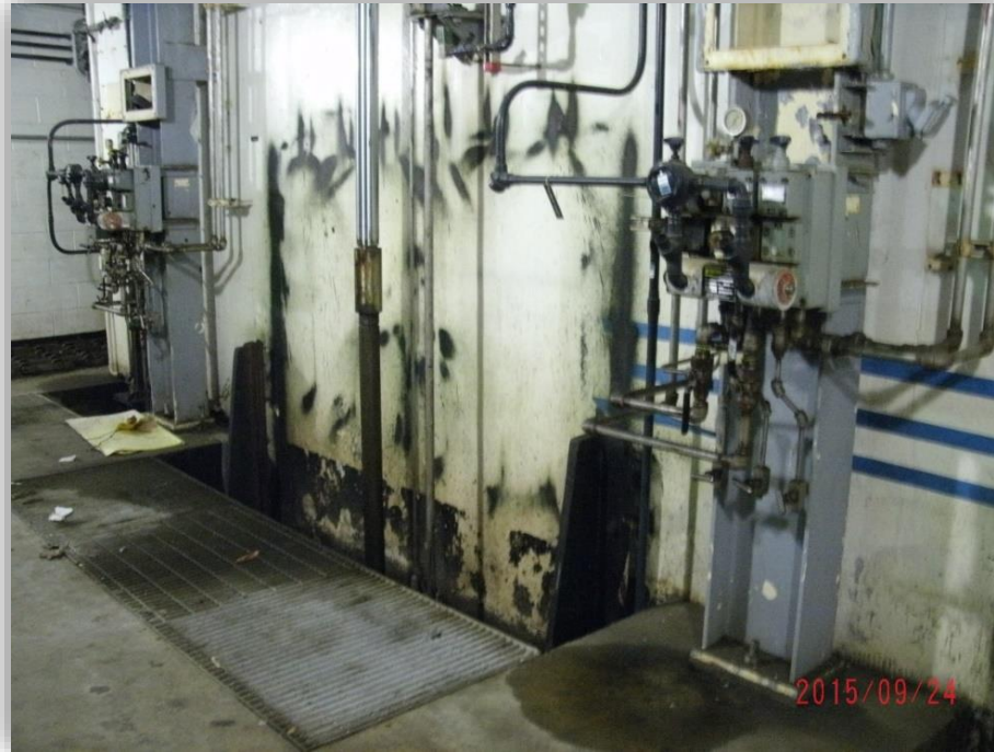
Influent Wet Weather Gate to be Replaced
