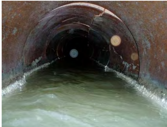
Sewer Rehabilitation Needed to Address Pipeline Defects
