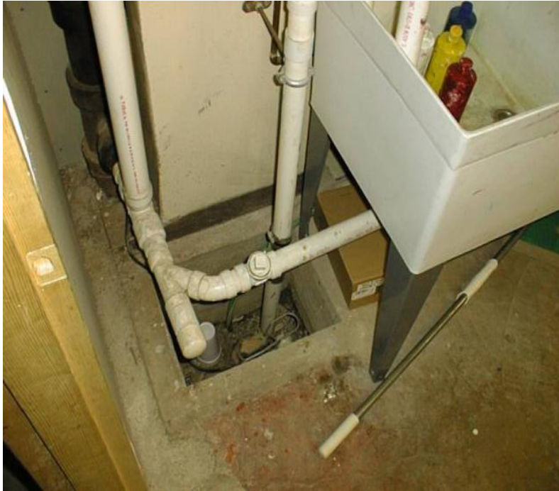
Sump Pump Direct Connection to Sewer
