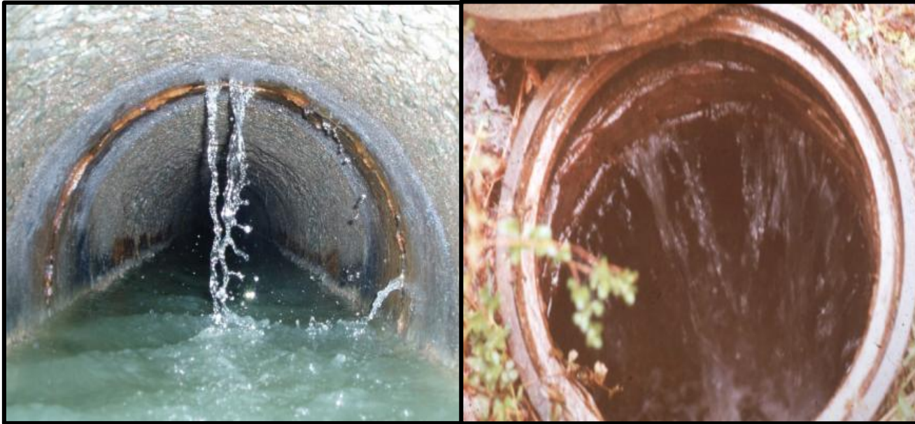
Infiltration (Groundwater via physical defects)
