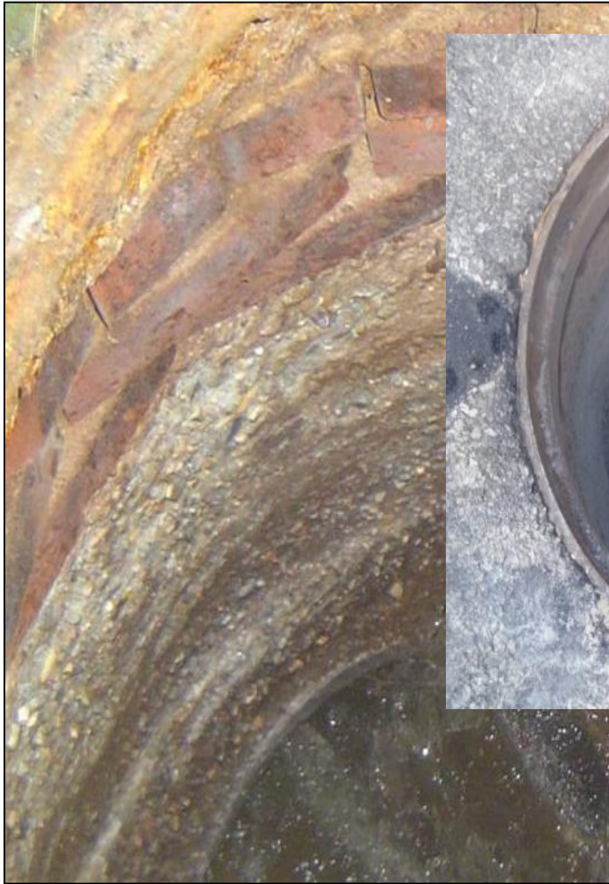
H 2 S Deterioration of Manhole
