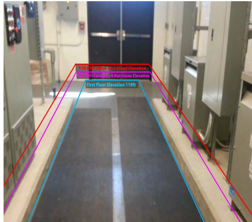
Interior South Side View First Floor Switch Gear Room
