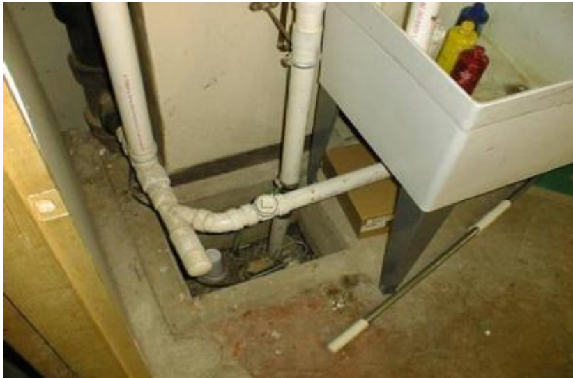
Sump Pump Inflow
