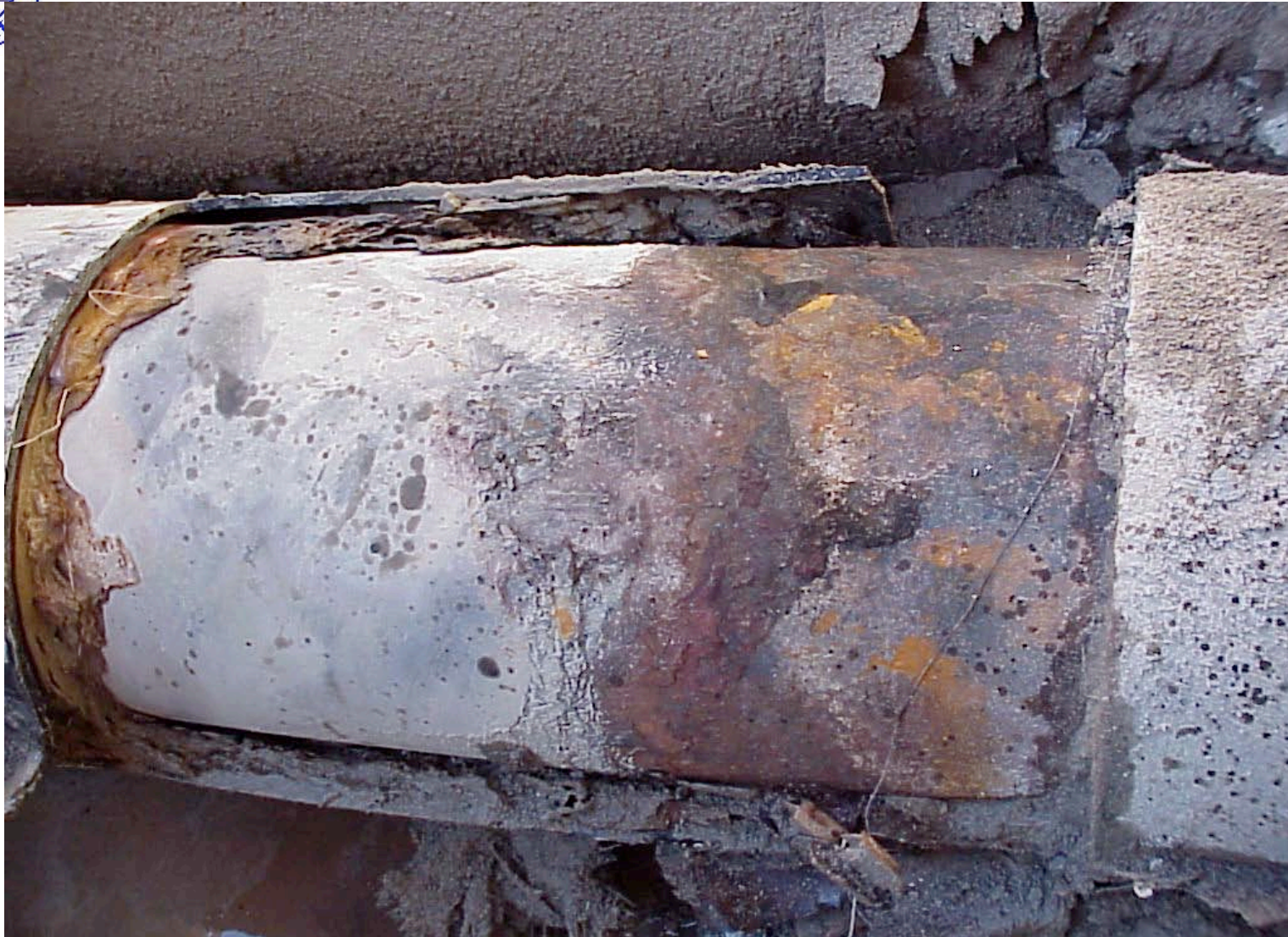
H1S/H1R Piping Failure
