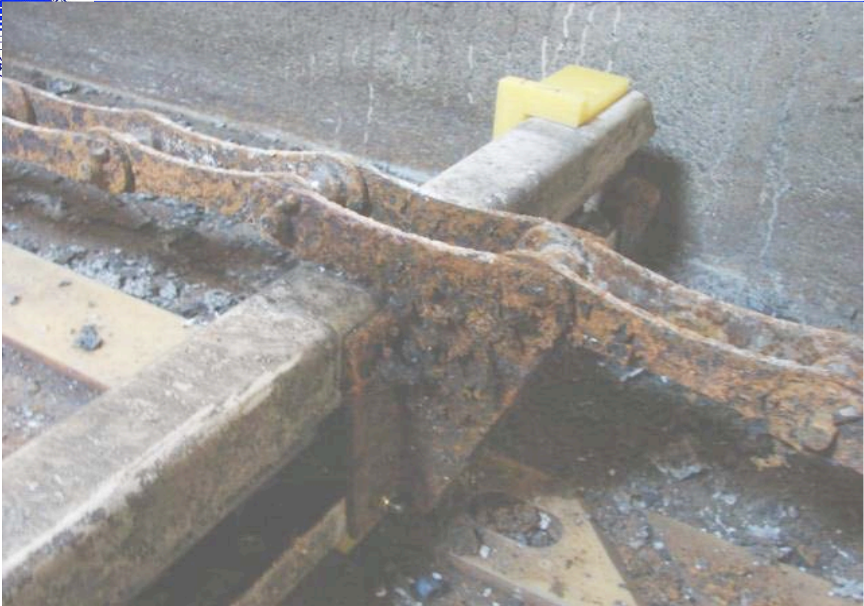
Significant Corrosion on Primary Chain (Typical)
