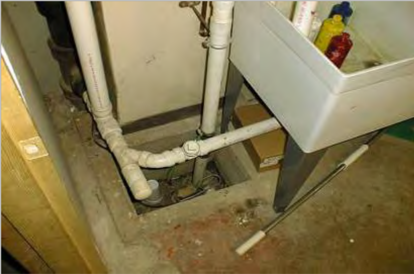
Sump Pump Inflow
