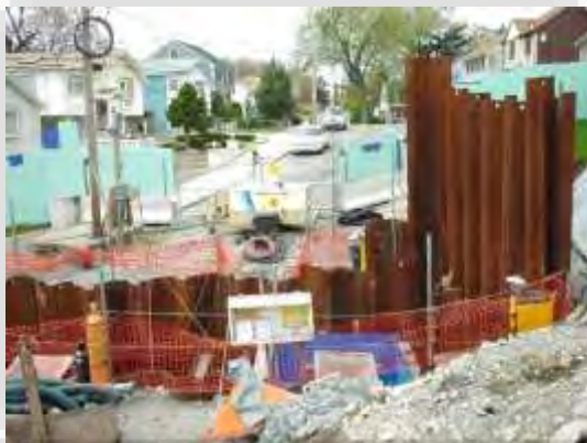
2002 Rehab. to New Haven Street Drop Chamber and Wellesley Extension Relief Sewer
