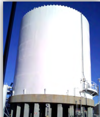
1,000 Ton Liquid Oxygen Storage
