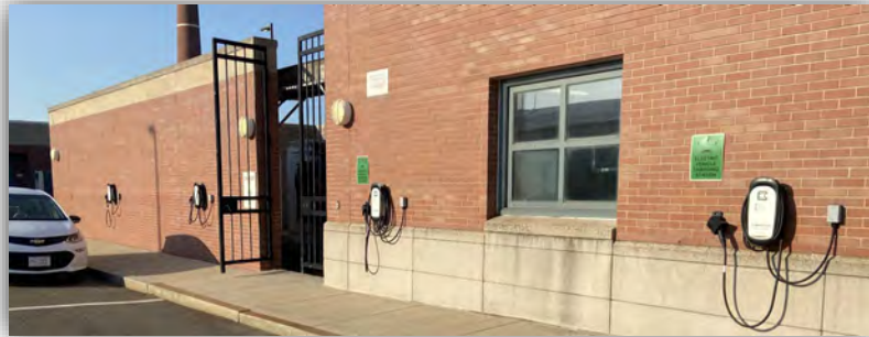
Existing EV Chargers
