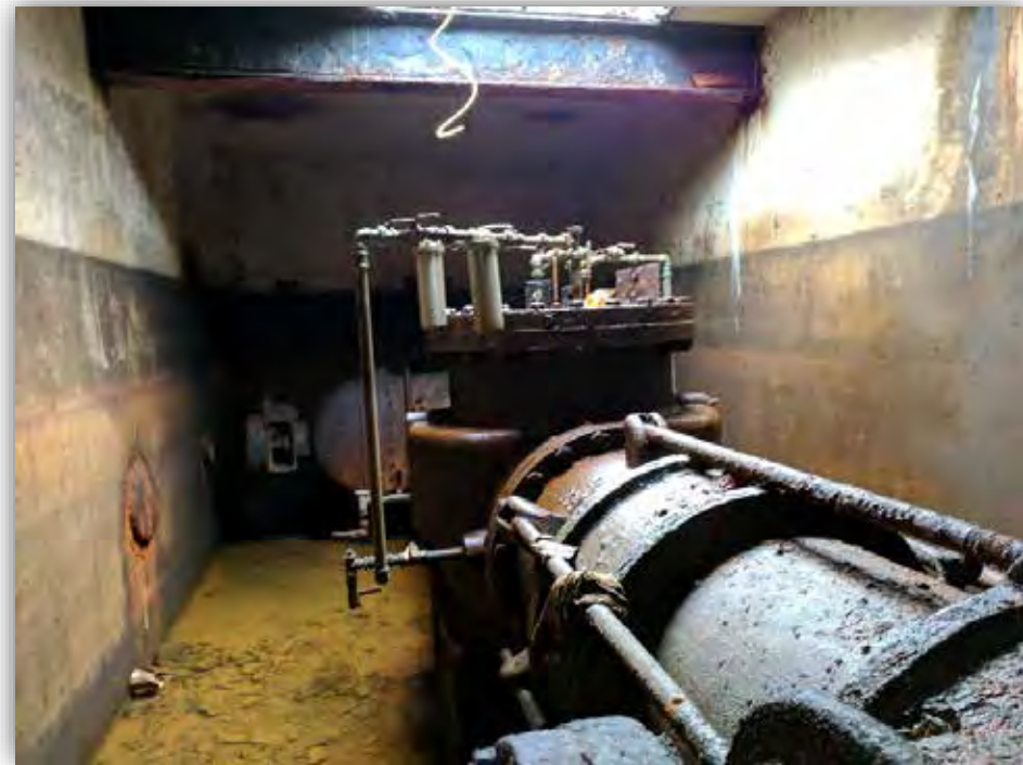
W16 Mystic Valley Parkway PRV Vault
