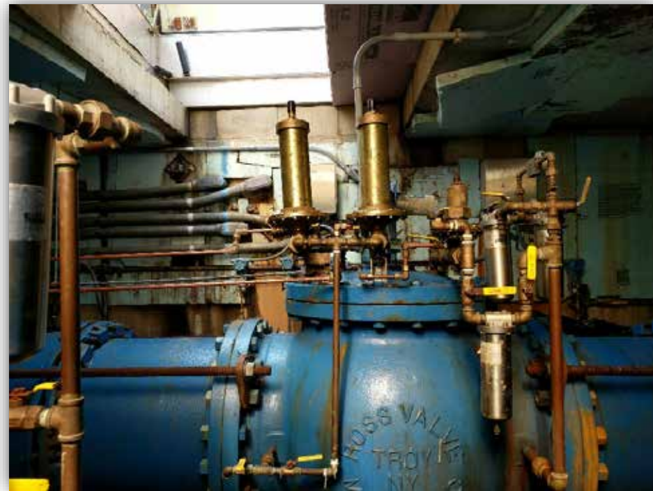
W14 Nonantum Road PRV Vault
