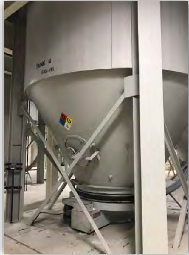
Soda Ash Silo
