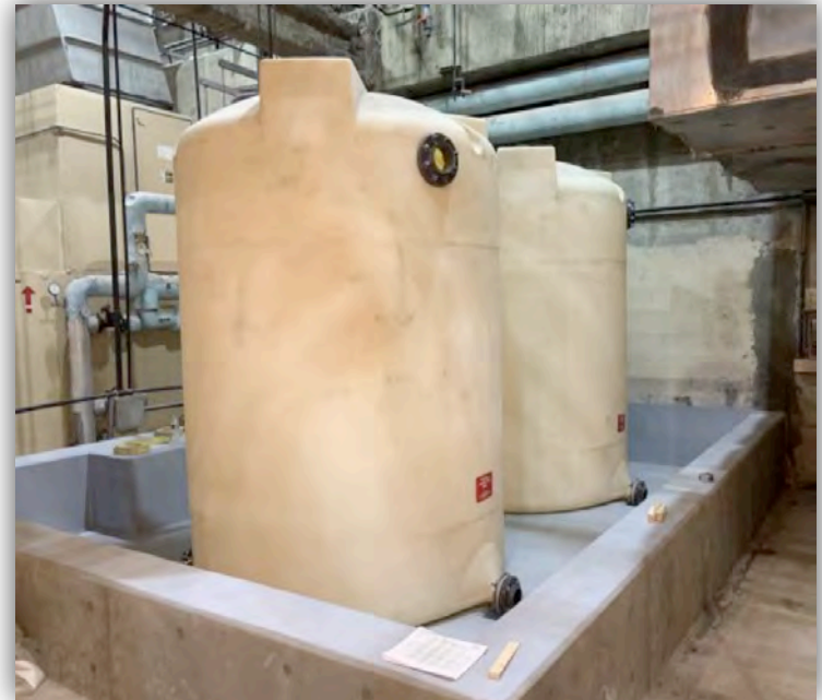
New Sodium Hypochlorite Tanks
