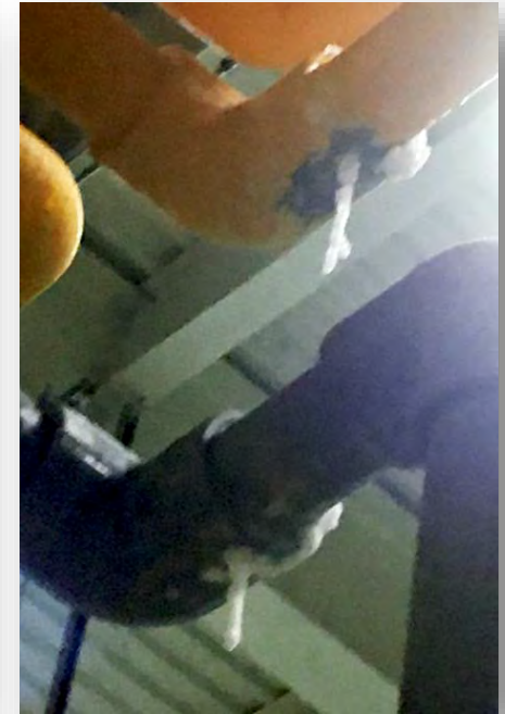
Sodium Hypochlorite Leak
