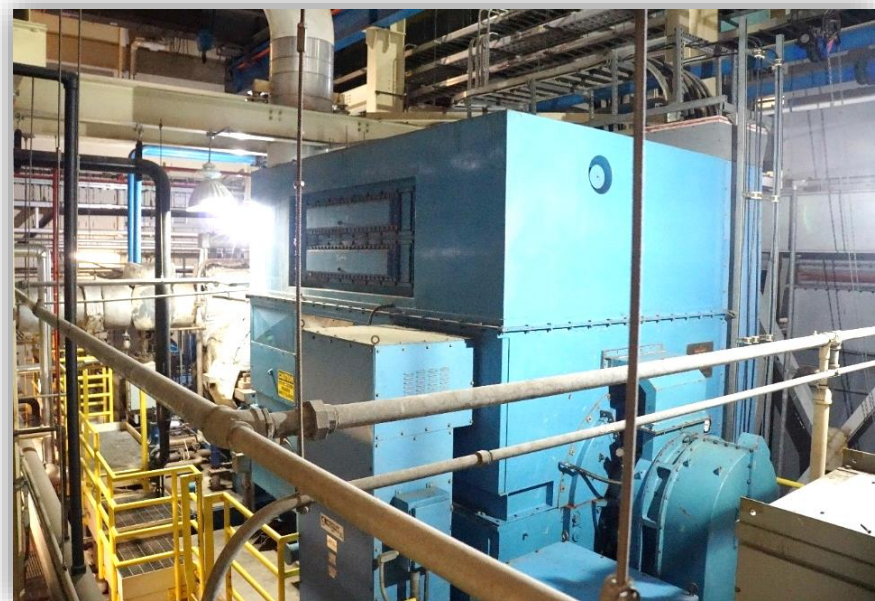
Steam Turbine Generator
