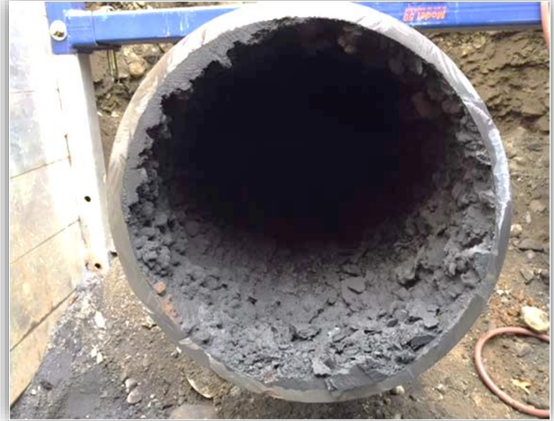
Section 24 20-inch Cast Iron Main St. James Terrace, Newton
