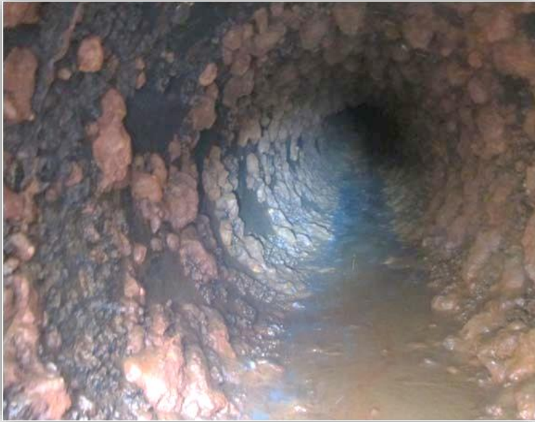
Section 23 36-inch Cast Iron Main Ward Street, Newton
