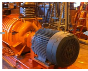
Biogas Booster Blowers
