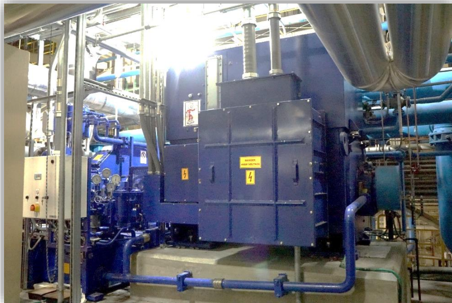
Back Pressure Steam Turbine Generator
