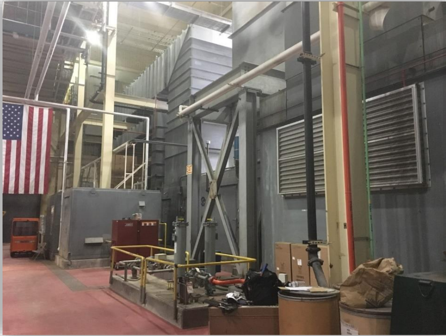
Combustion Turbine Generators
