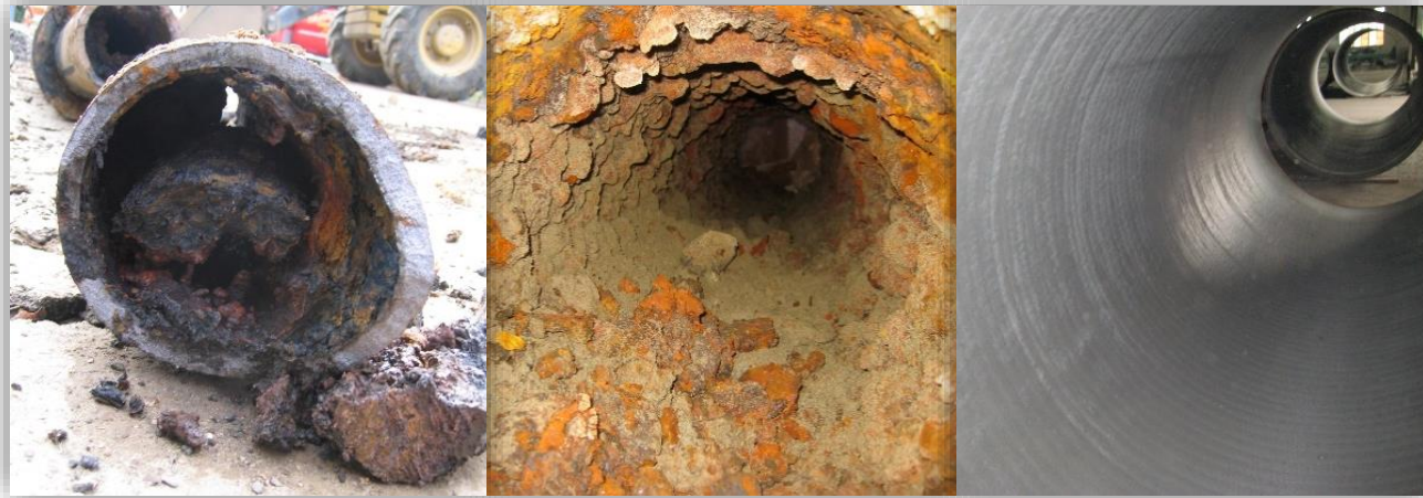
Unlined Cast-Iron Tuberculated Pipe
