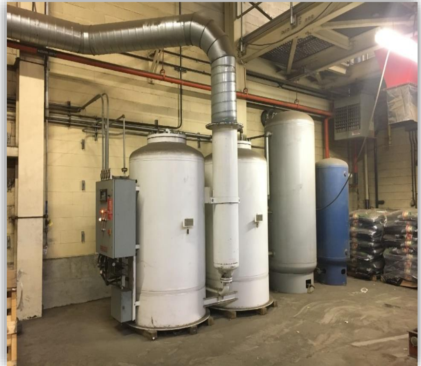
Nitrogen Purge Generator (fire suppression system)
