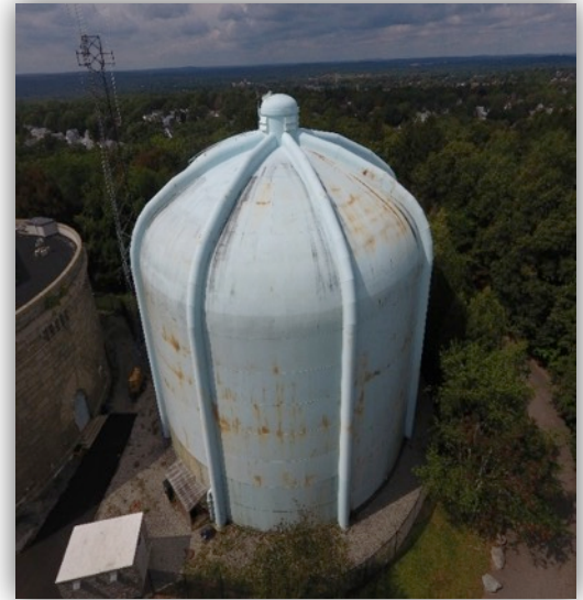
Bellevue II Water Storage Tank – West Roxbury
