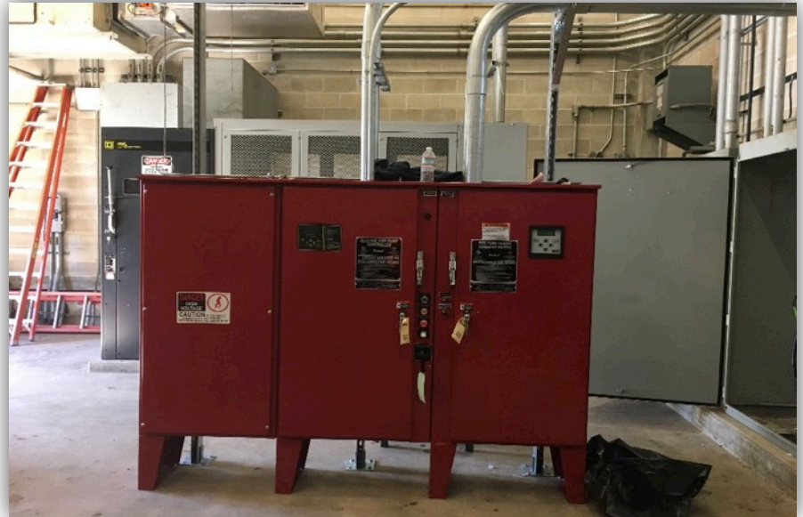
Newly Installed Nut Island Fire Pump Controller
