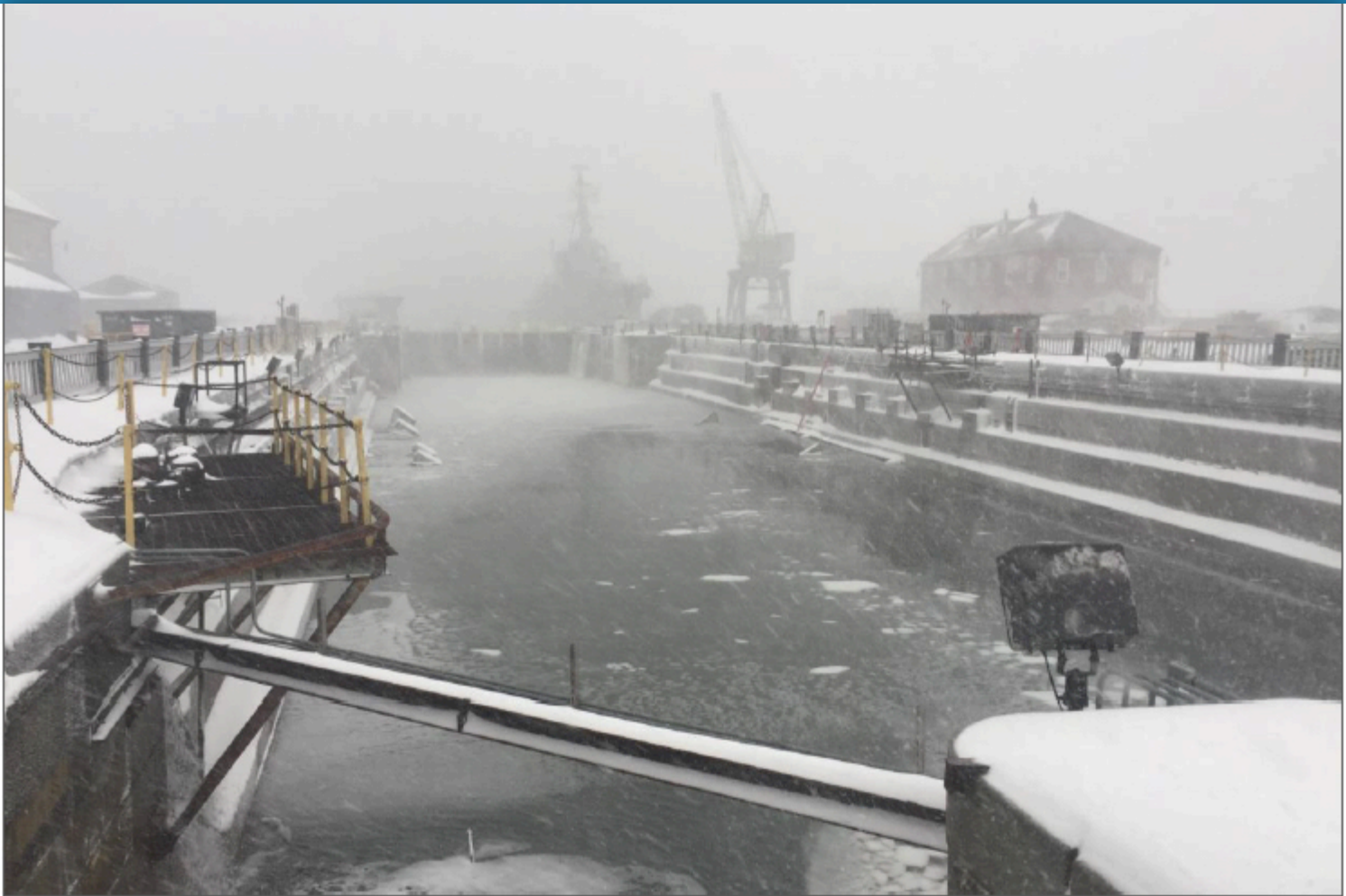
Dry Dock received 15 feet of water from overflow of caisson, overtopping and pump drains
