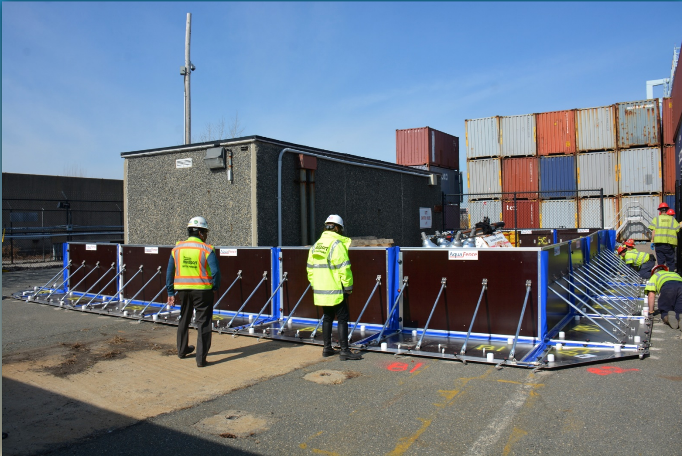
Protecting electrical equipment
