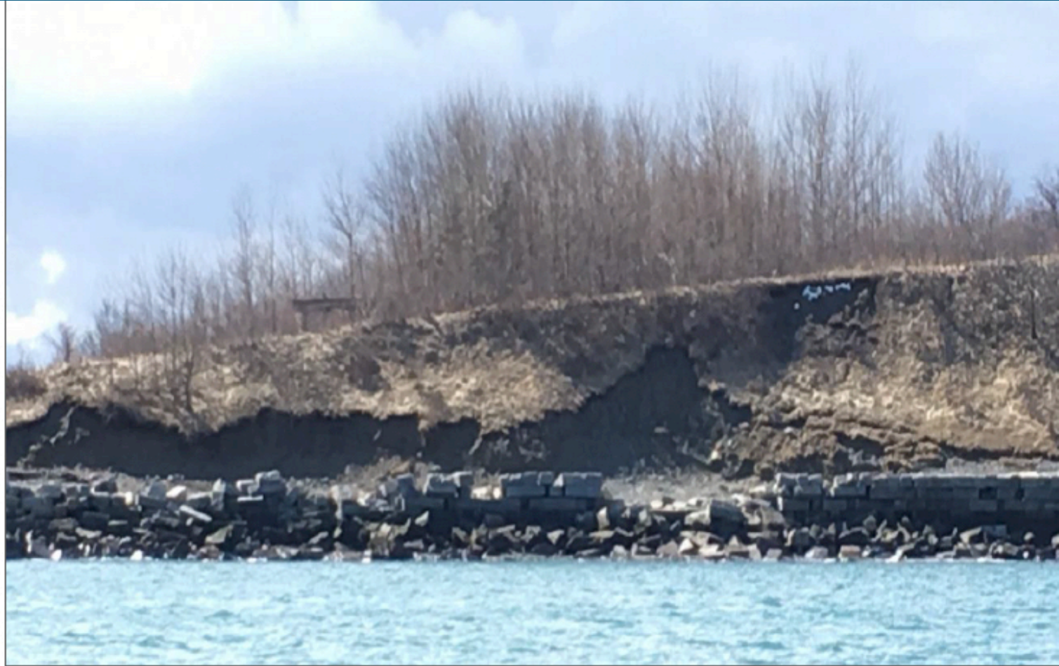
Looking southwest, showing continued damage to historic seawall and erosion of bluff that protects cemetery
