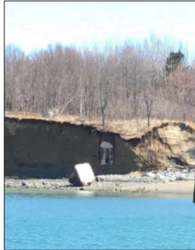
Looking east, showing perched doorway and tunnel entrance associated with Fort Standish coastal defense installation
