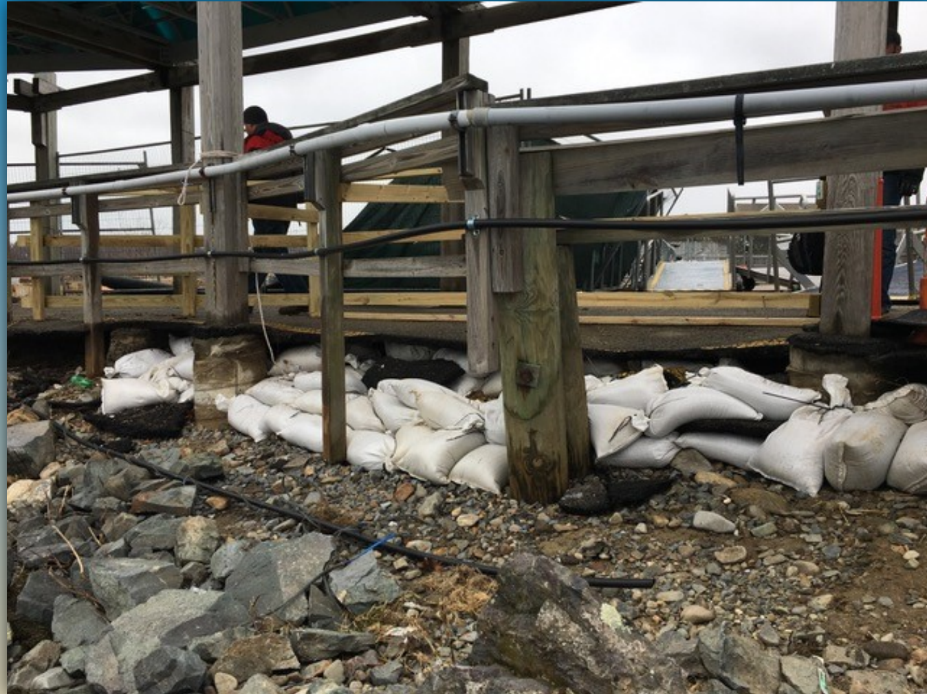
Undermined revetment and walkway
