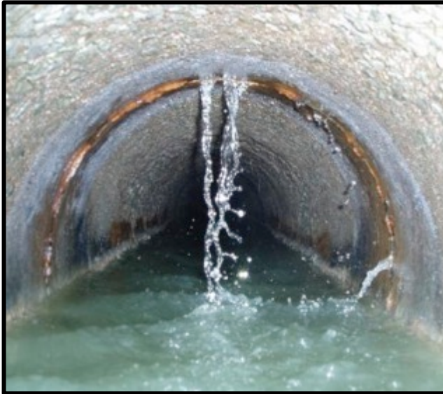
Infiltration (Groundwater via physical defects)
