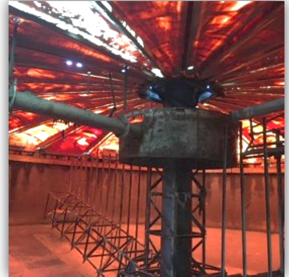
GT 5 Center Cage failure caused lower structure (rake arms) to lift off GT floor
