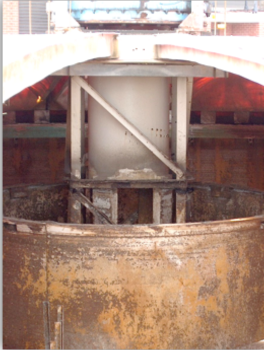
Undamaged Center Cage
