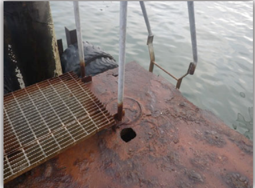
Prior to summer of 2015 repair
