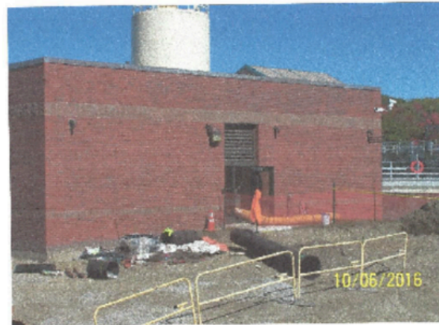
Chemical Building pressure release/vents at the south end
