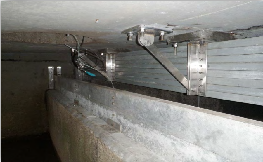
Underflow baffle (floatables control) Behind existing overflow weir
