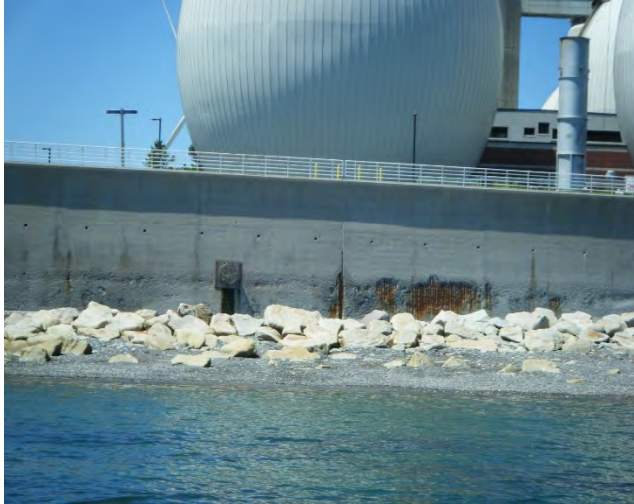
Concrete deterioration and exposed reinforcing steel
