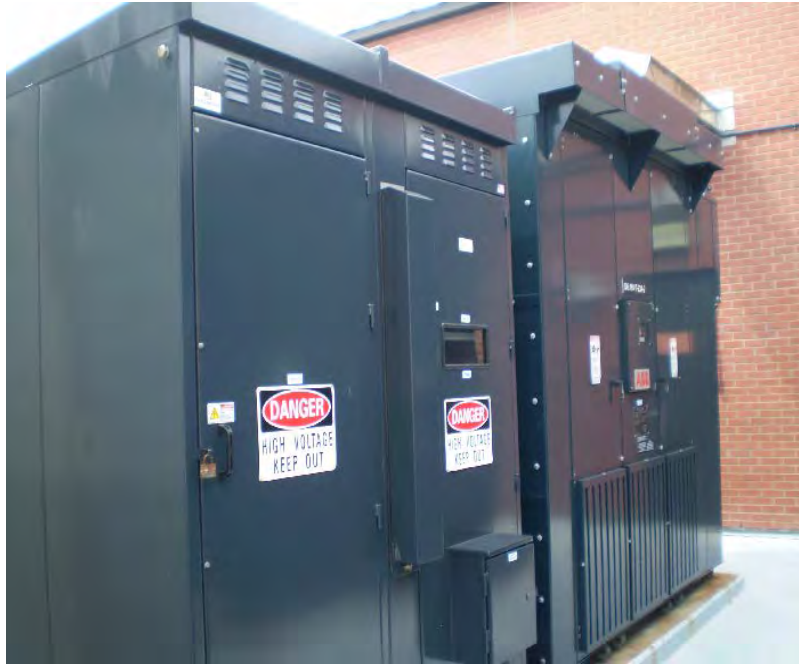
Figure 1 – Typical Electrical Substation
