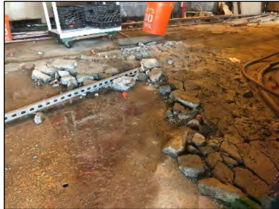
Topping Slab Crumbling in Odor Control Room
