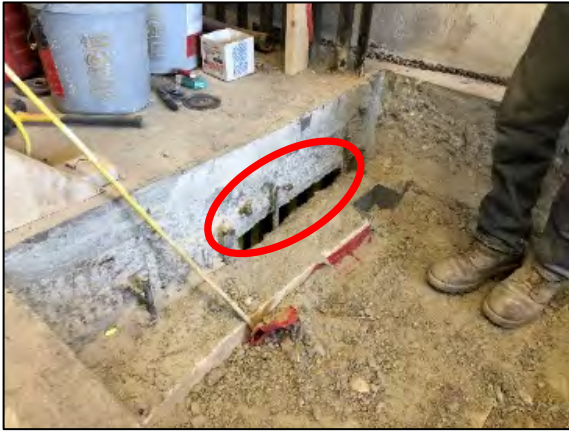
Contractor chipped into mezzanine level
