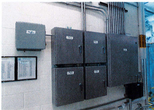
BACport Control Cabinets
