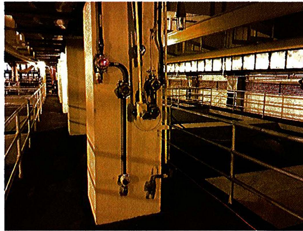
Gas Sensors Located on Operating Floor
