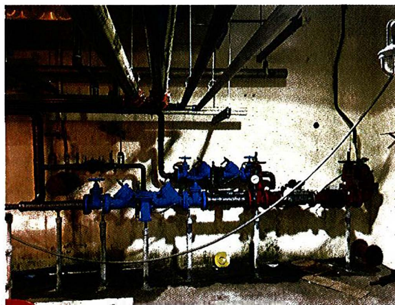
Backflow Preventer and water for new domestic service
