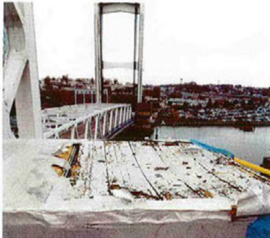
HVAC insulation breaking down
