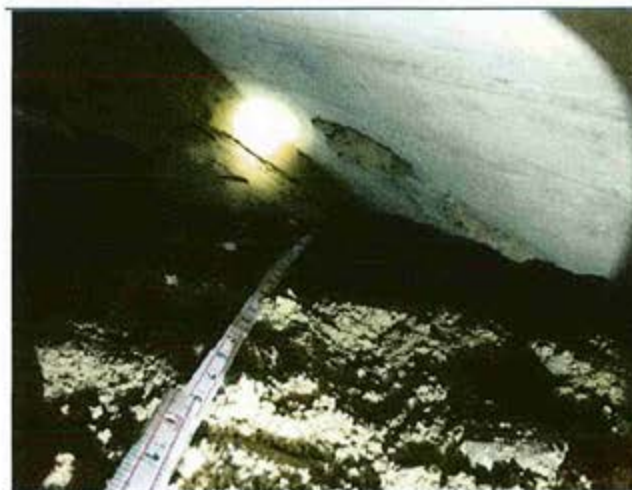
Photo shows the void under the right parapet wall.
