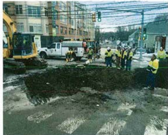
Pavement damage at River and Seyon
