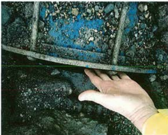
Pipe appears to have pulled out of coupling
