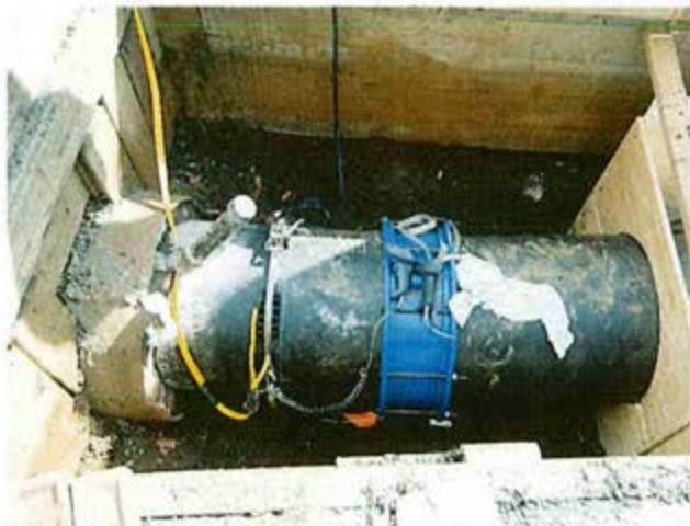
Typical coupling locations with flex restraints being fused on (before concrete block poured)
