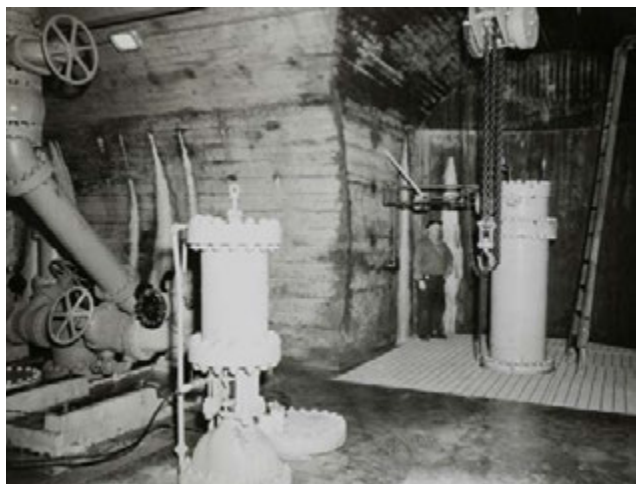
1959 photo of valves in Shaft 9 Chamber
