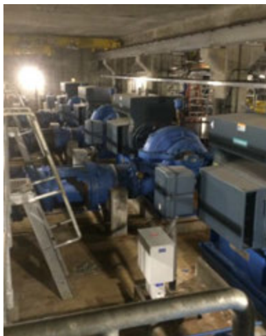
Chestnut Hill Emergency Pump Station
