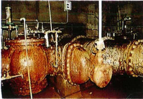
Shaft 8 Isolation valves and PRVs
