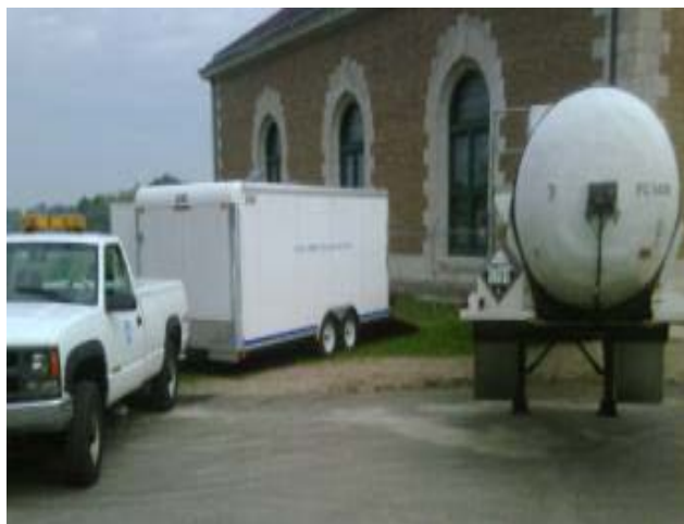
Mobile disinfection unit and chlorine tank at Gillis Station
