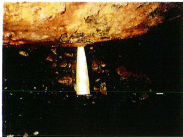
Plugged Leak Prior to Cap Weld
