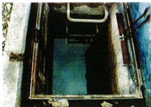
Ground water in top of Shaft Chamber
