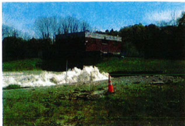
Shaft 5 Break. May 1, 2010
