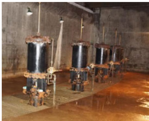
Shaft 7 valve actuators
