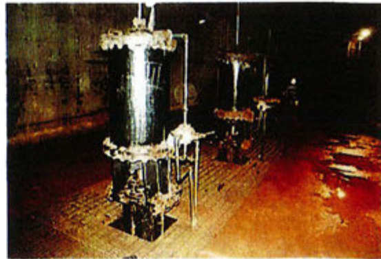
Shaft 7 Hydraulic Valve Operators
