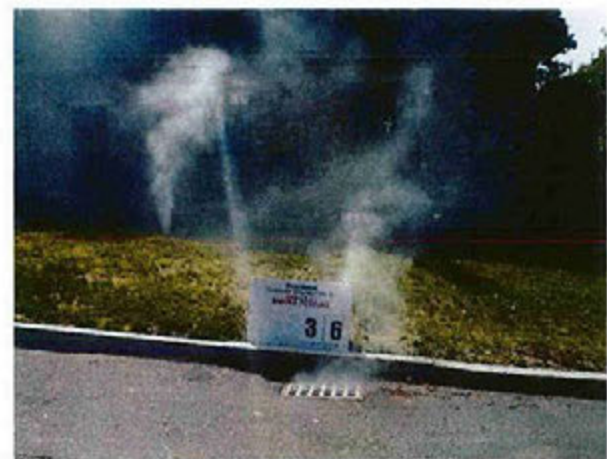
Smoke Testing of Sewer Confirms Catch Basin and Open Service Connection Clean-Out are Inflow Sources
