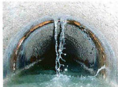
Infiltration in a Sanitary Sewer
