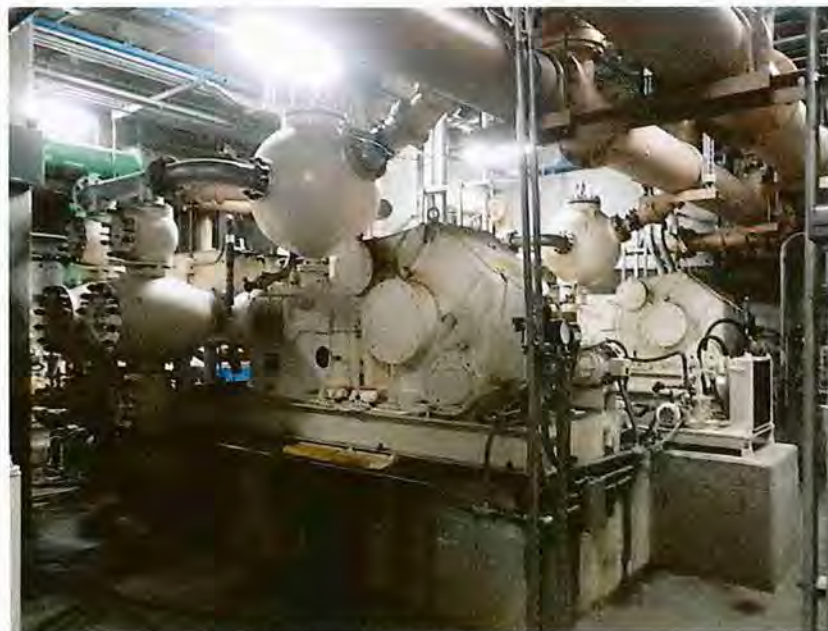
Existing Abel Pumps
