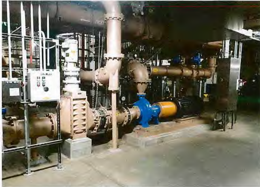
Prototype Pumping System
