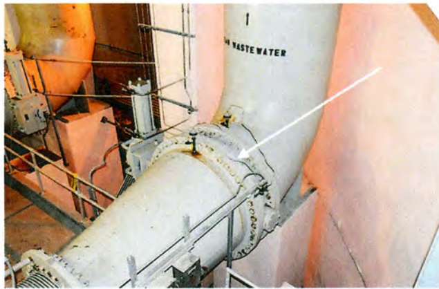
Lower 60-inch Butterfly Valve in NMPS
