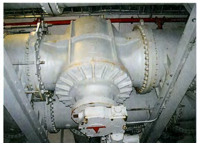
48-inch Plug Valve on WTF Force Main
