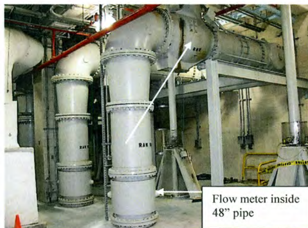
Check Valve and Flow Meter in WTF
