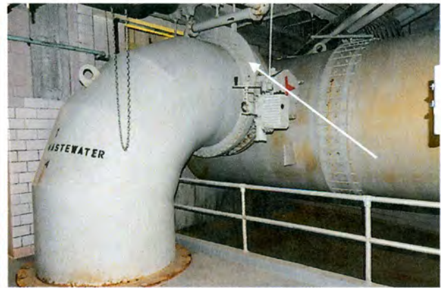
Upper 60-inch Butterfly Valve in NMPS
