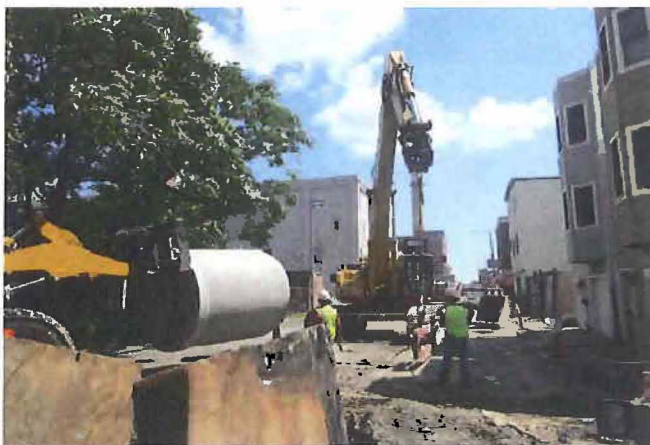
Figure 2: 72-inch storm drain installation in East First Street (Reserved Channel Contract 3B)
