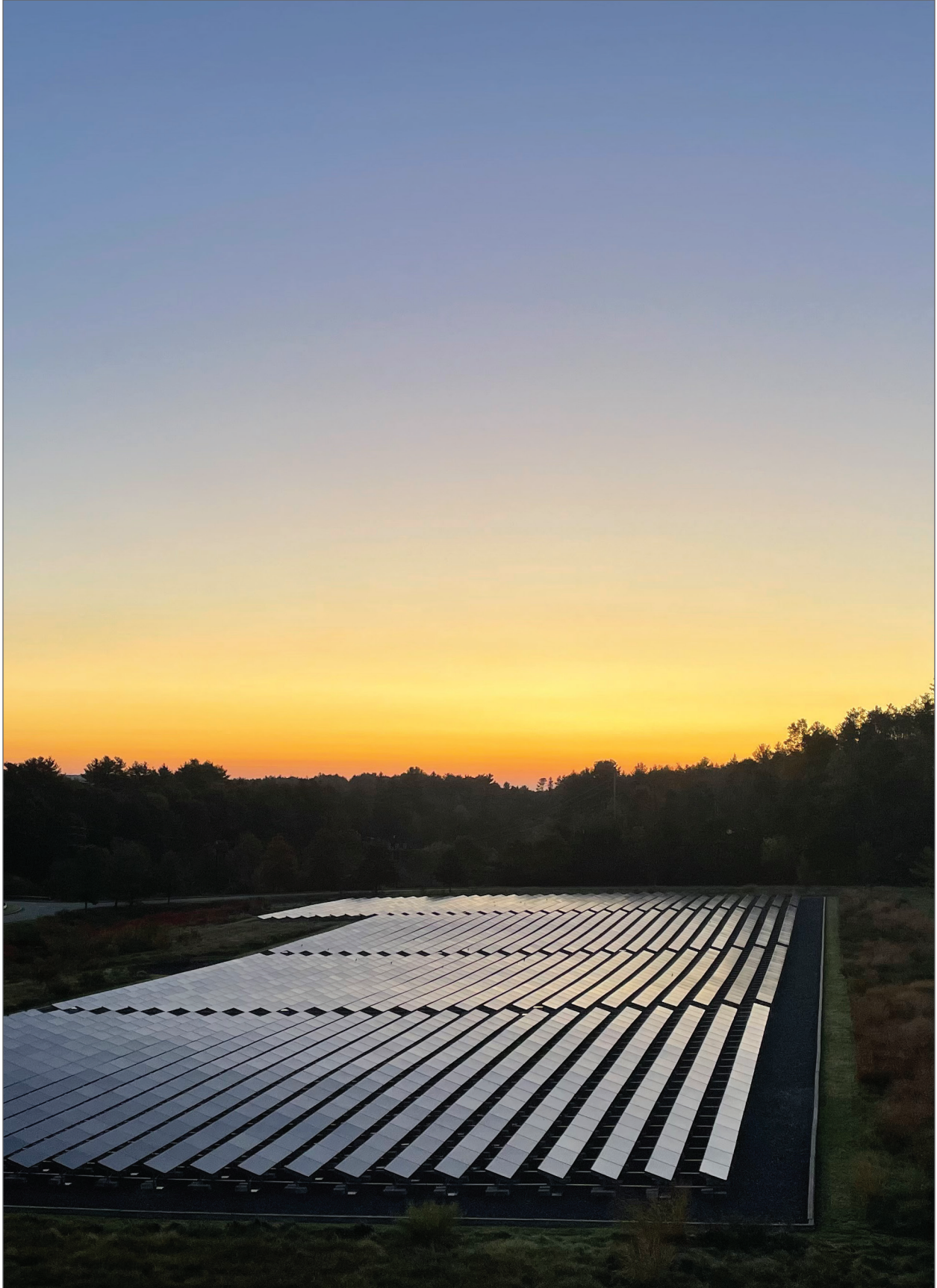
Solar panels at Carroll Water Treatment Plant
