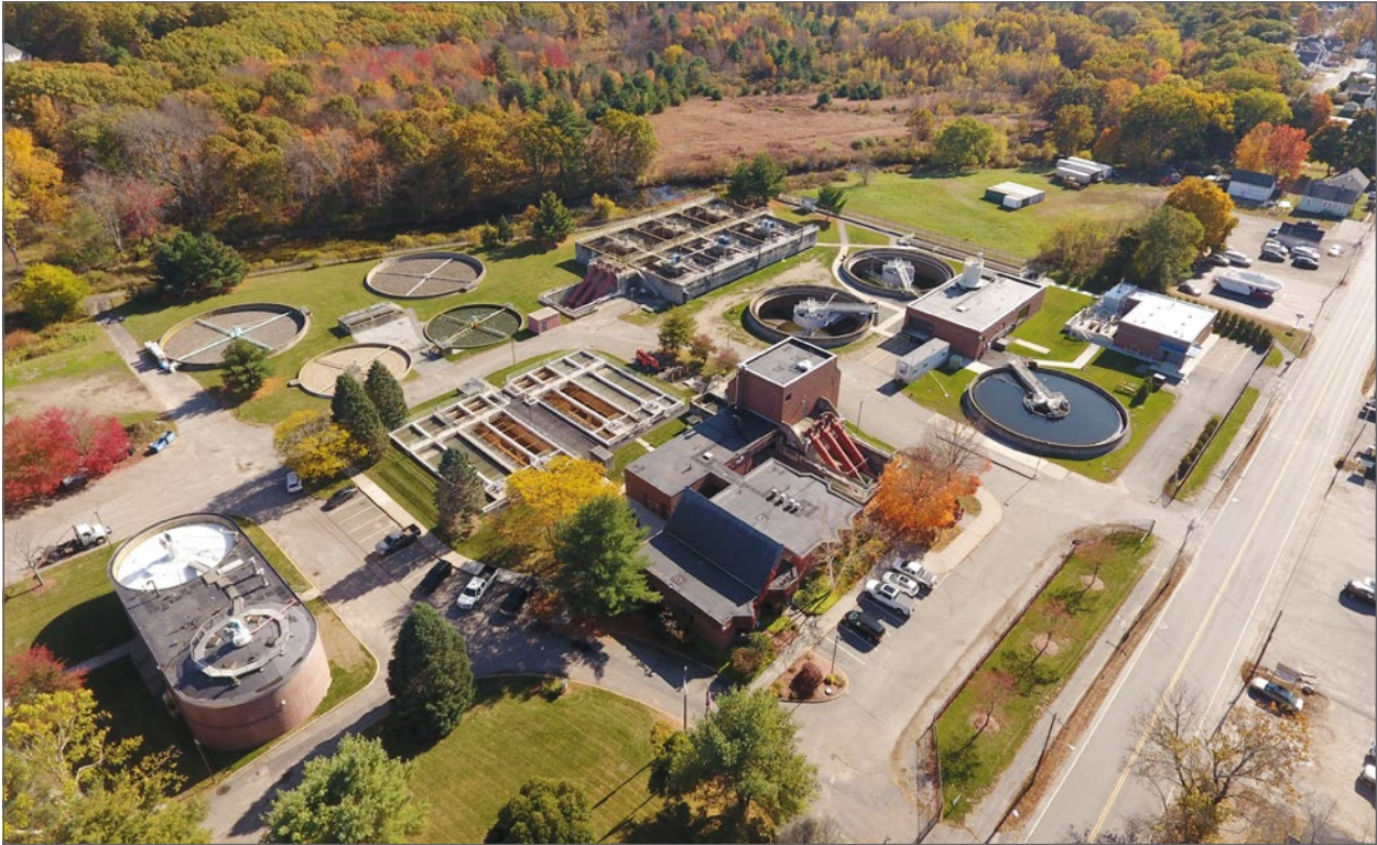
Clinton Wastewater Treatment Plant
