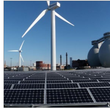
Wind turbines and solar panels at the Deer Island Wastewater Treatment Plant
