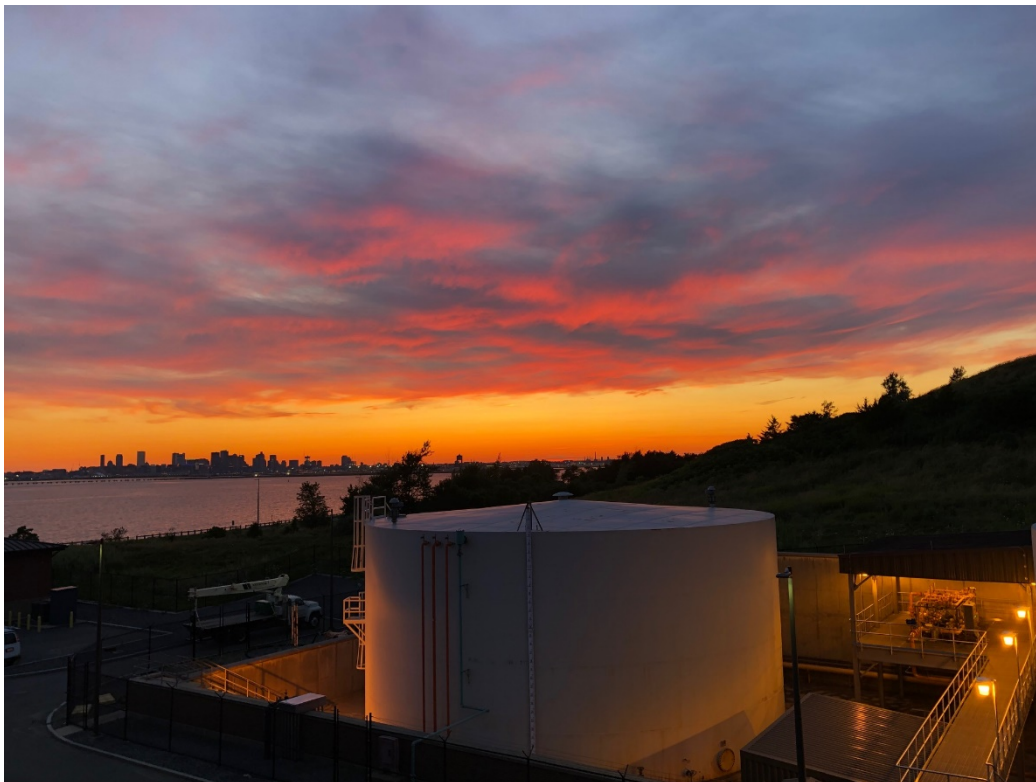
Deer Island Treatment Plant Thermal Power Plant
