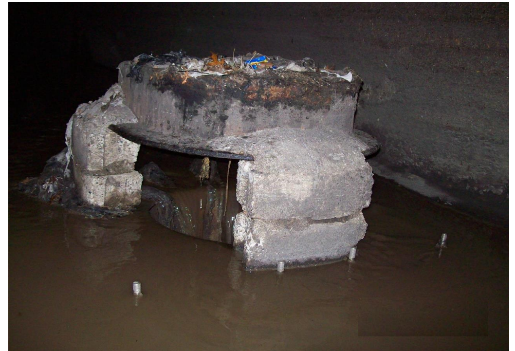
Connection to interceptor at SOM01A
