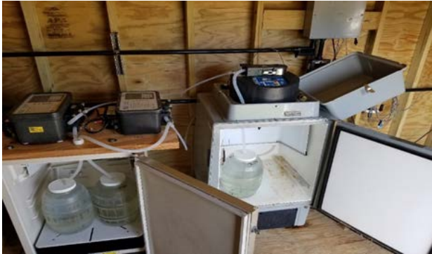
Figure 3: Auto samplers for NPDES and Local Limits at the Clinton Wastewater Treatment Plant
