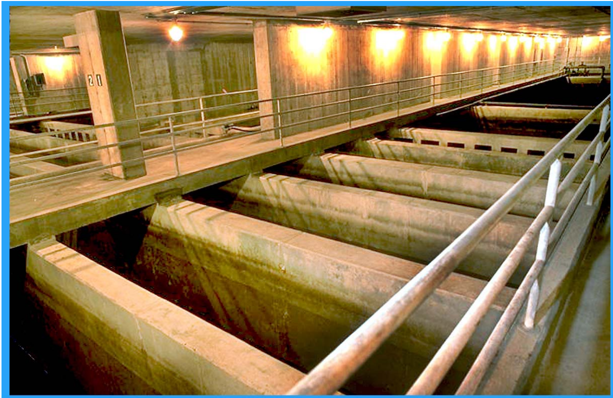
Below Ground Detention Tanks at Prison Point CSO Facility
