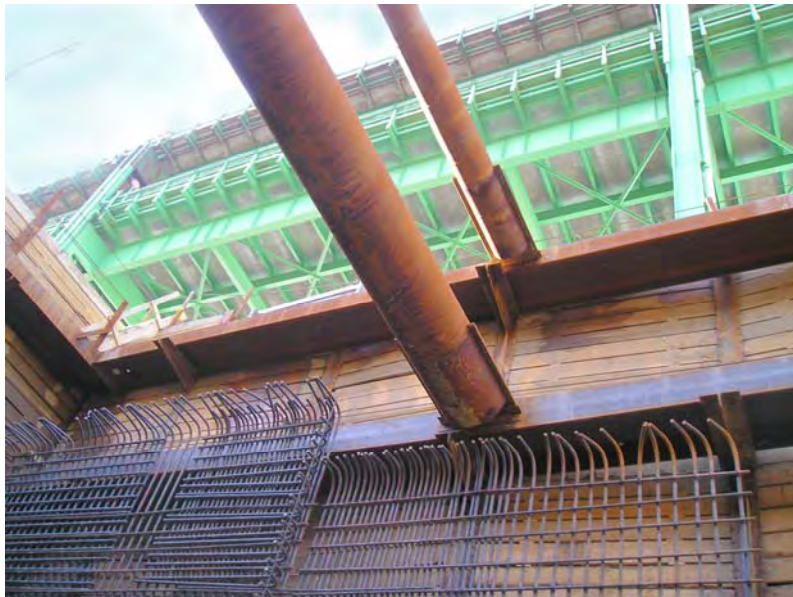
View from bottom of BOS019 storage conduit trench; Mystic River Bridge above
