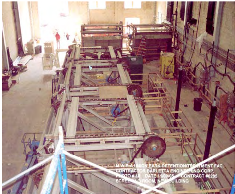
New screening room, two coarse screens (rear) and four fine screens
